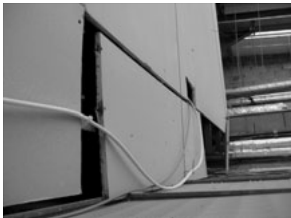
Effective compartmentation must be reinstated following refurbishment
