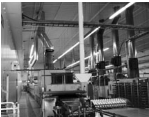
Ductwork should be carefully designed and properly installed
